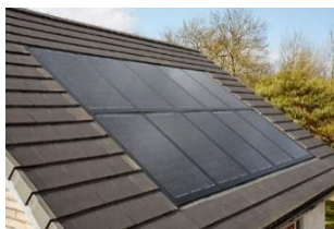
PV panels flush with roofing tiles
